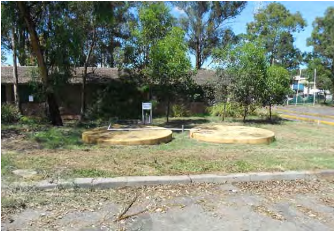
Photograph 6 - Recycled water tanks
